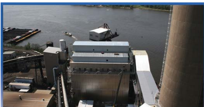
A baghouse was recently installed at Dairyland's John P. Madgett power station to enhance particulate matter capture.
